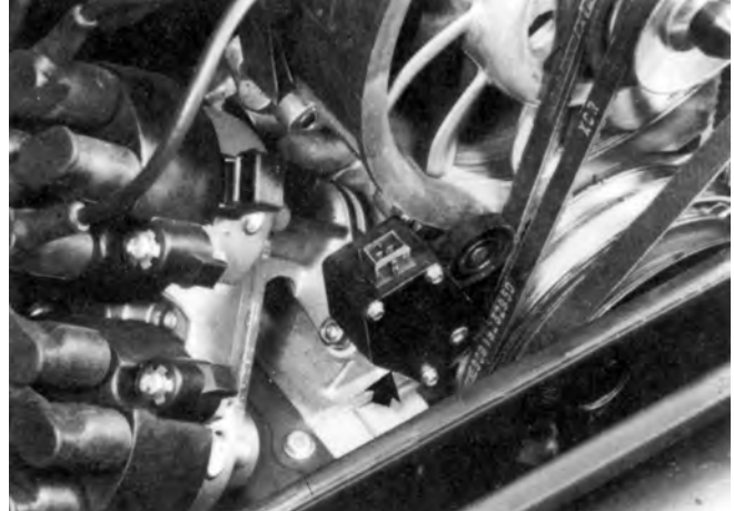
The engine blower drive belt is controlled by a drive belt monitor (arrow).
